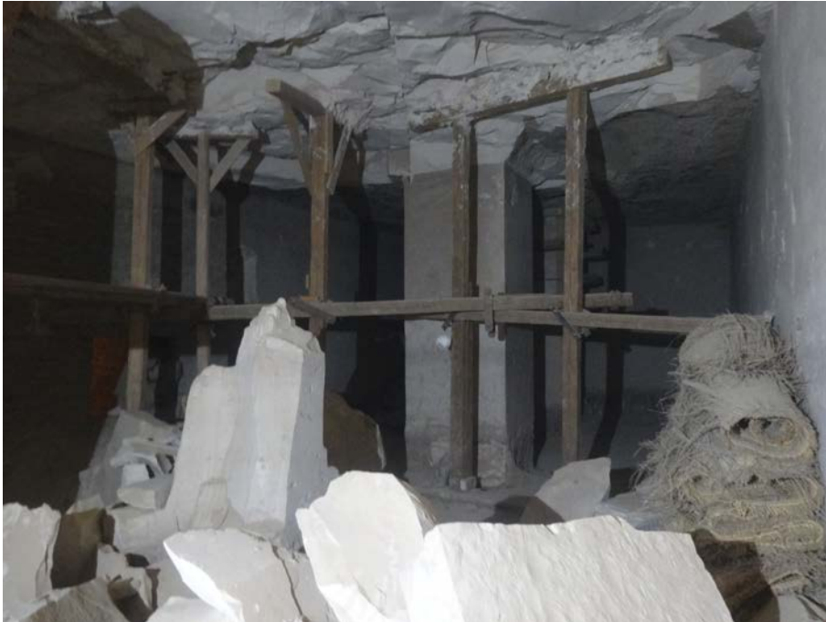
Fig. 11. Ceiling and collapsed pillar in KV 17 Jc.
